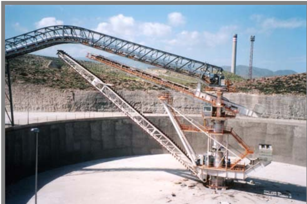
Coke/Coal Handling System – Carboneras Plant - Holcim (Spain)
